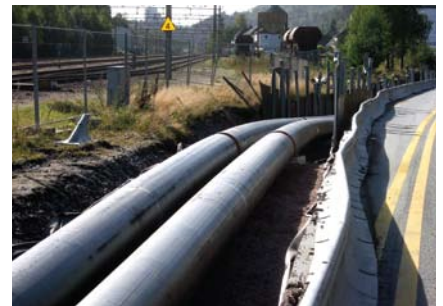
District Heating - Norway
